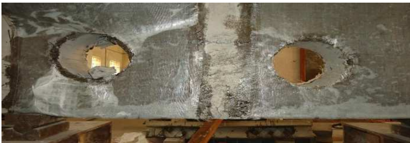
FIG. FLEXURE CRACK AT THE MIDPOINT OF THE BEAM
