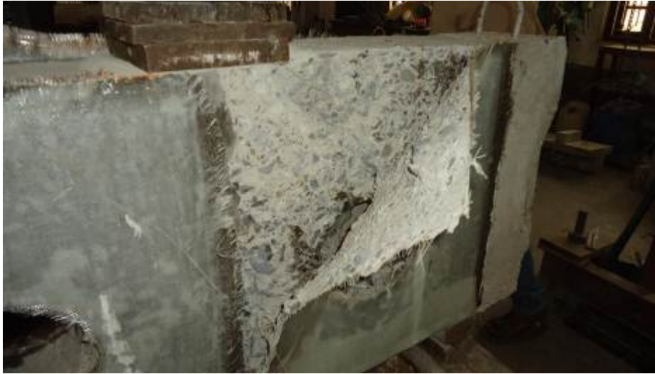
FIG. DEBONDING OF GFRP
