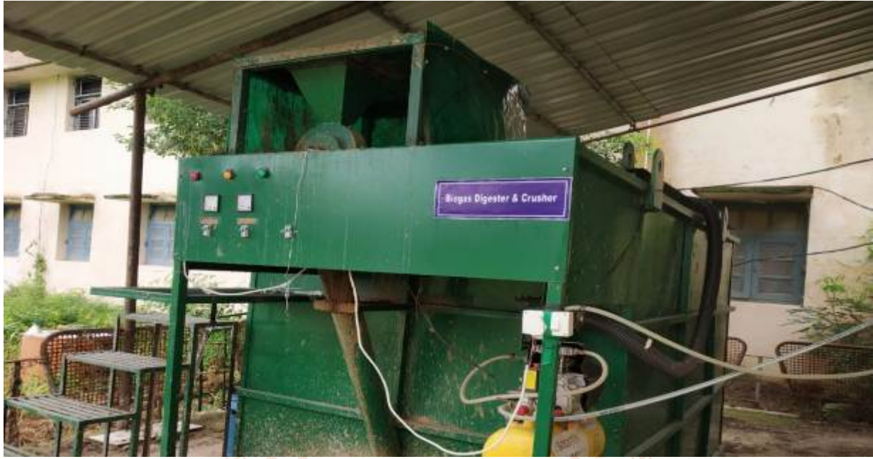
Figure 3 Biogas Digester and Crusher
