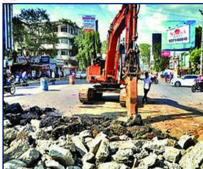
Fig -5: Demolition of Infrastructure Project in Nashik (Trimbak Naka to Ashok Stambh Road)
