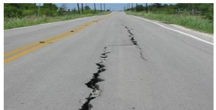
Fig-1 longitudinal cracking
