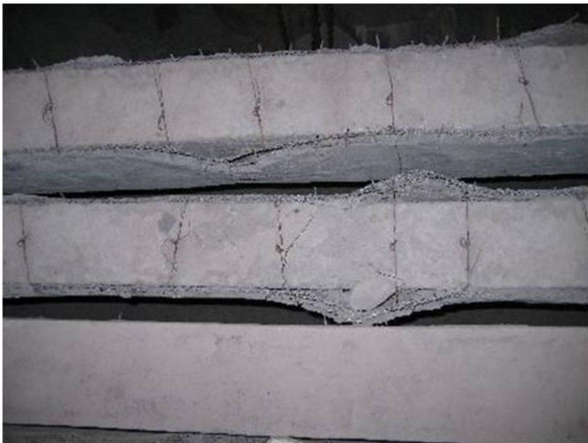
FIGURE 3.12: FAILURE OF BEAMS
