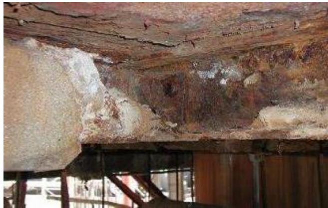
Fig 8 Crack development in concrete structure due to fire.
