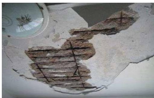
Fig. 7 Spalling of concrete
