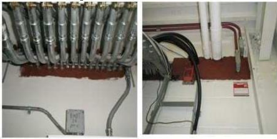
Fig. 13 Fire penetration protection system
