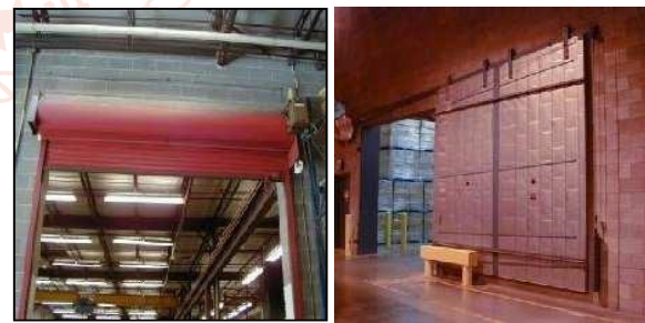
Figure 12 Fire Door (a) Vertical ("Roll-Up") Fire Doors (b) Horizontal ("Sliding") Fire Door
