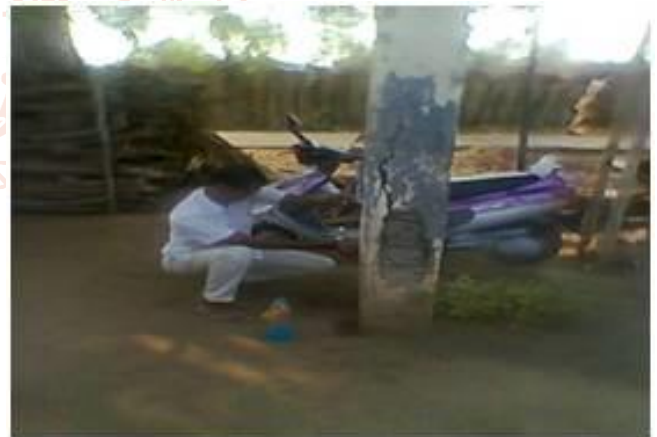
Fig.3.4 Half Cell Potential Difference Test being conducted on Column of the Water Tank
