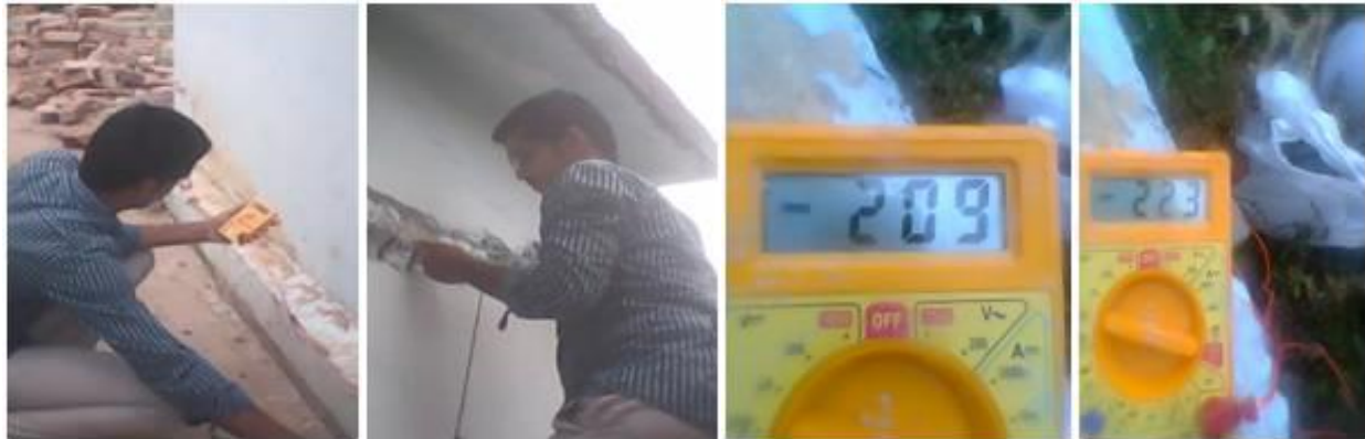
Fig 4.1 Half Cell Potential Difference test being conducted on the Ration Shop building
