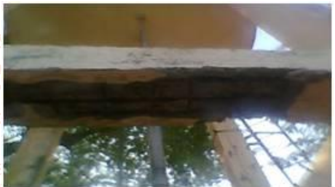
Fig.3.3 Image of the Spalled Brace of the Water Tank
