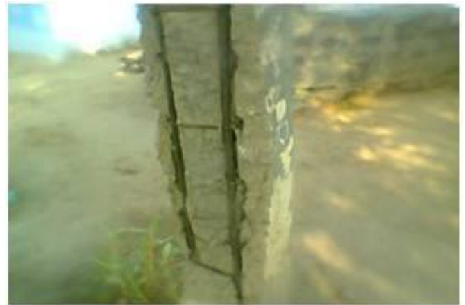
Fig.3.2 Image of Spalled Column of the Water Tank
