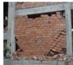
a) Infill Compression and Shear Damages
