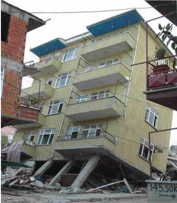
Fig: Partial collapse of RC frame building with masonry infill walls in Yingxiu during Wenchuan earthquake.
