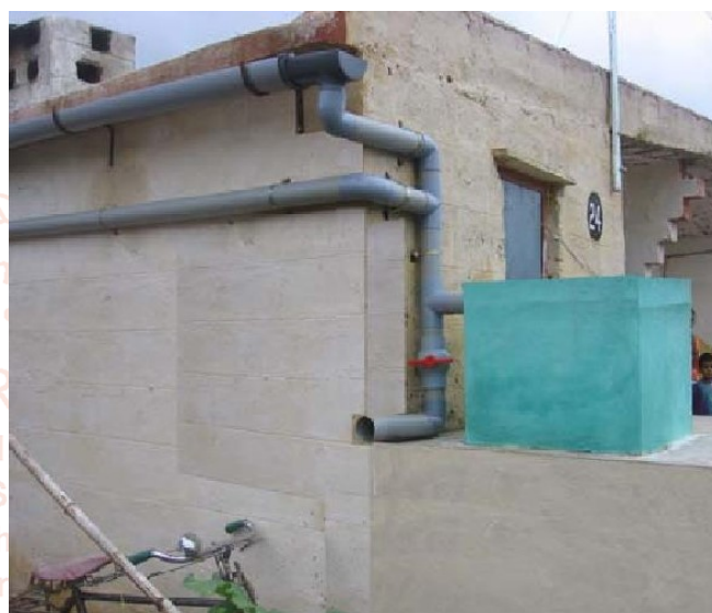
RAINWATER HARVESTING SYSTEM IN JAMUI
