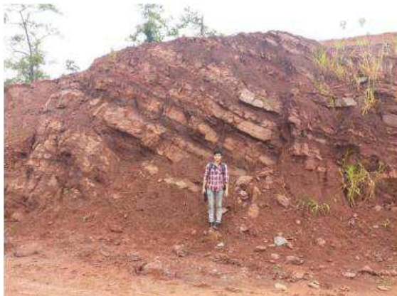
Figure (3.1.c) Outcrop photo near the left abutment of Upper Keng Tawng dam axis
