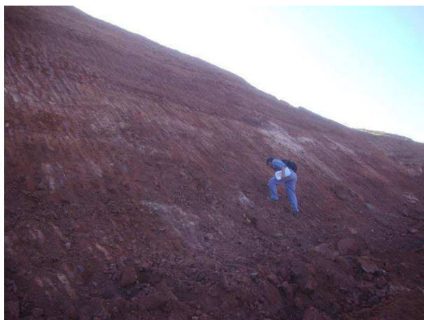
Figure (3.4.a) Slope cutting near the right abutment of Upper Keng Tawng dam axis
