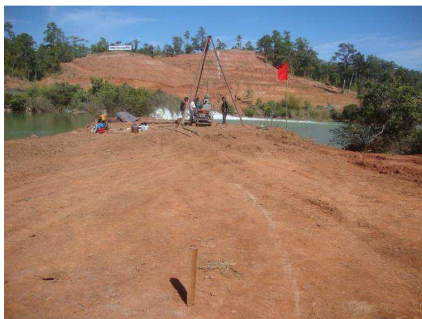
Figure (3.4.b) Diamond Core Drilling at right abutment of Upper Keng Tawng dam axis
